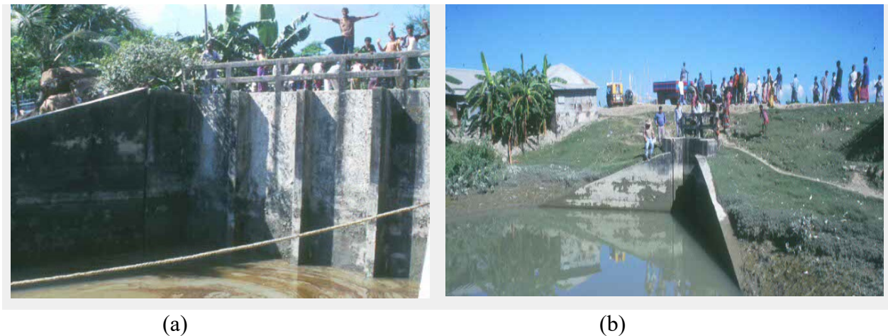
Figure 5.6 (a) One of the 28 sluice gates; (b) an coastal embankment in Sandwip Island ( Murdoch University, 2000)
